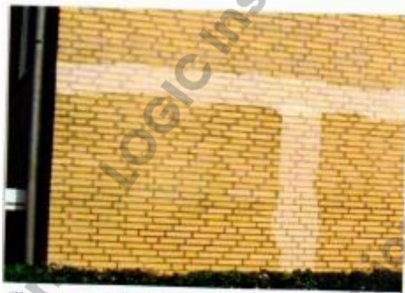
White smooth traces on top of overlapping silicon treatment on exterior after silicone treatment.
